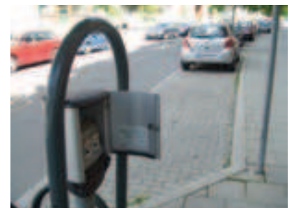
Electric car charging points
